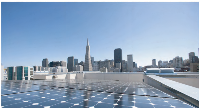
View of Luminalt's Solar Installation, Courtesy of SunPower Corporation
