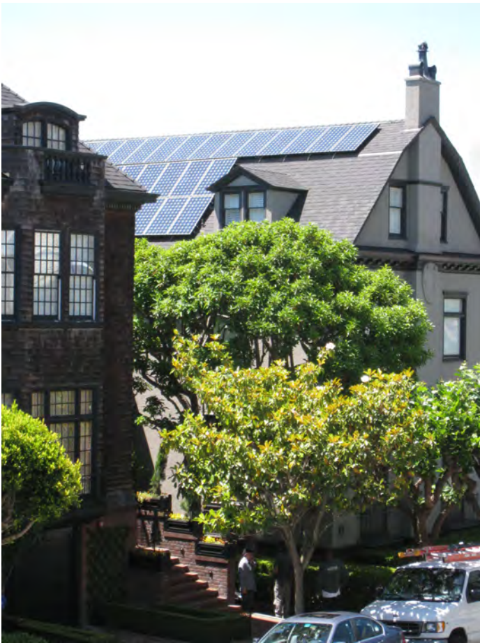
Solar Installation in Presidio Terrace by Luminalt
